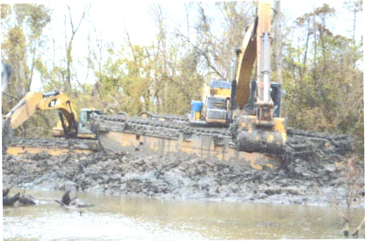
Figure A: This photo was taken by Dean Wilson during the monitoring trip in the Basin on December 7, 2018. This photo was taken approximately 1.5 miles east of Flat Lake Pass. Approximate coordinates 30.08572778, -91.41138889. Figures A-C depict active construction in the area and a lack of erosion or sediment control measures in place.
