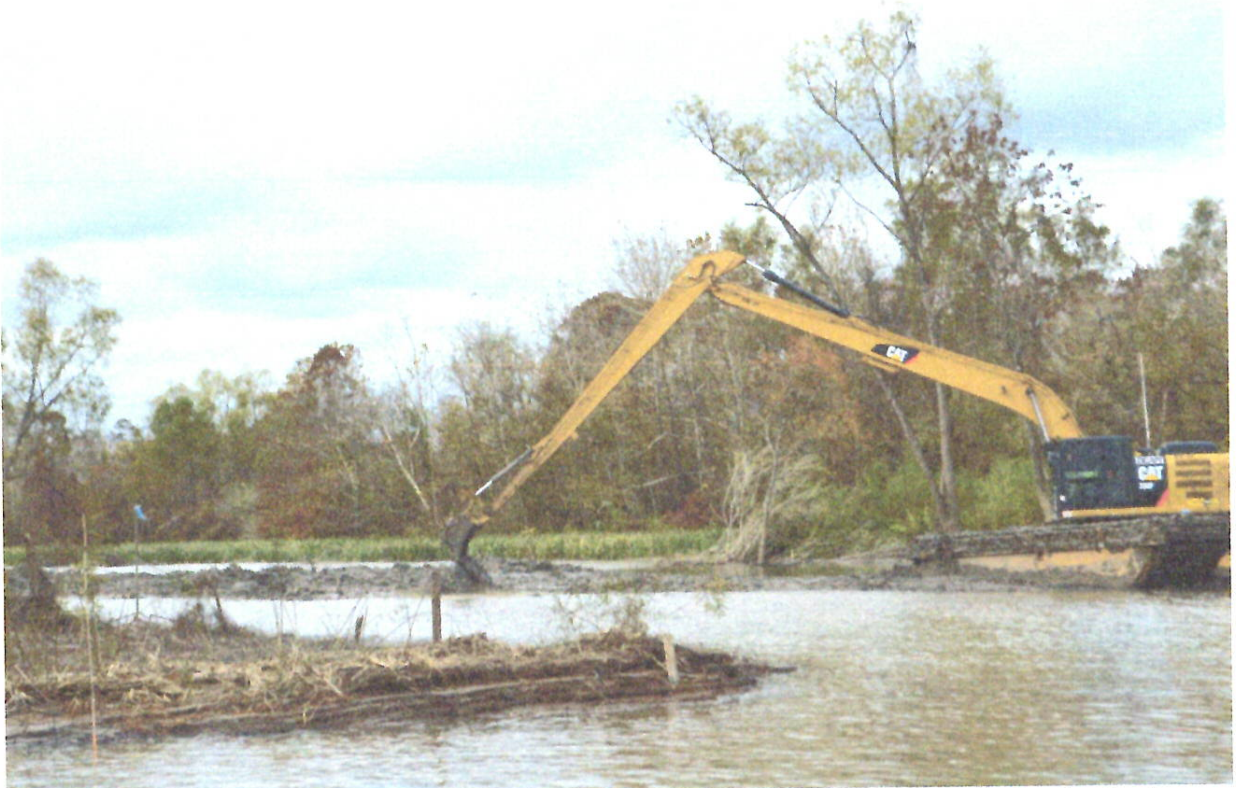
Figure B: This photo was taken by Dean Wilson during the monitoring trip in the Basin on December 7, 2018. This photo was taken in the same location as Figure A. This photo depicts active construction in the area and again, a lack of erosion or sediment control measures in place.
