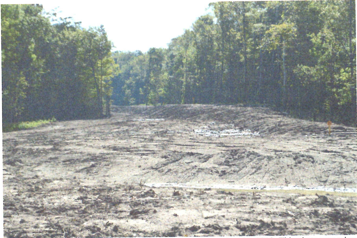
Figure G: This Photo was taken by Dean Wilson on September 20, 2018. This photo was taken facing southeast along the pipeline right-of-way at approximately 30.11311944, -91.54972222. This photo depicts an existing spoil pile on the south side of the pipeline right-of-way, and pipeline markers on top of the spoil pile.
